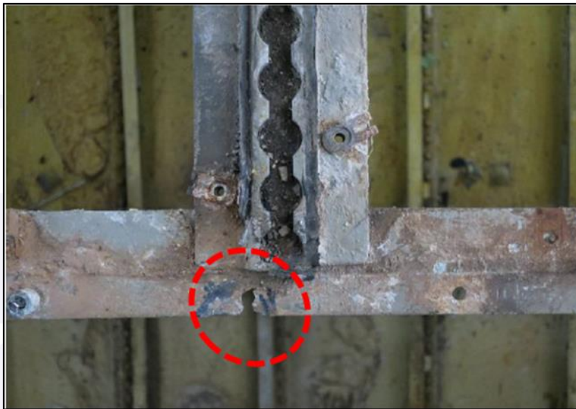
Figure 39 - Penetrating corrosion on the structural element securing the floor.
