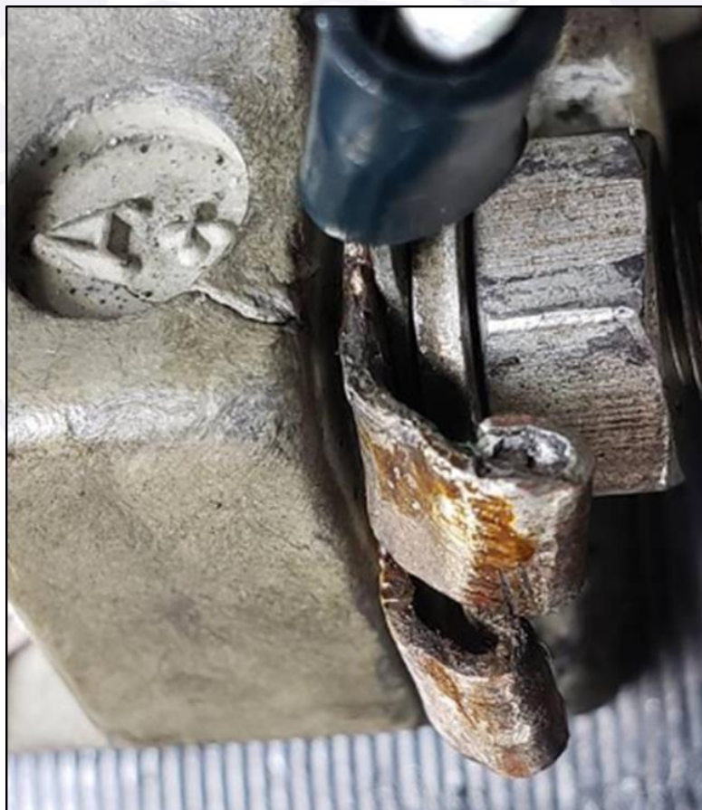
Figure 18 - Deformation of a contact washer on the terminal A+ of the Starter-Generator No. 2 .
