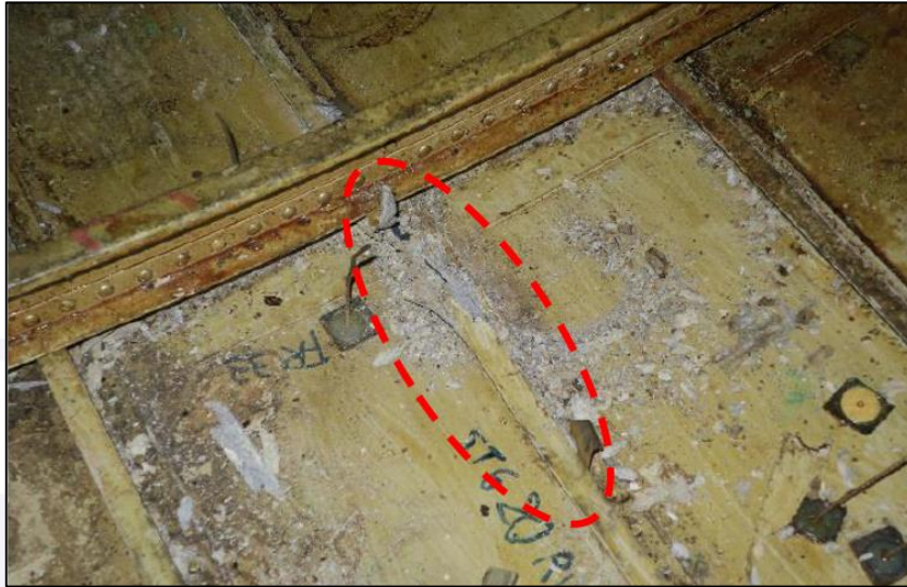
Figure 36 - Stringer 20RH, near frame 33, showing severe corrosion.
