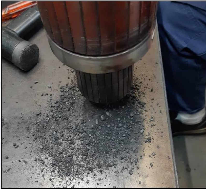
Figure 25 - High amount of metallic dust present on the rotor of the generator.
